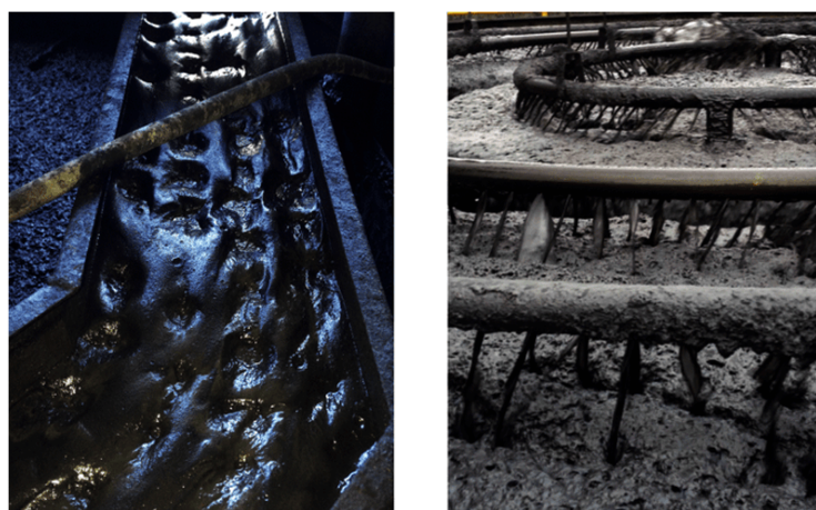
Figure 20 Plugged/blocked the wash water tray and wash water distributor ring pipes due to the poor quality of clarified coal water
