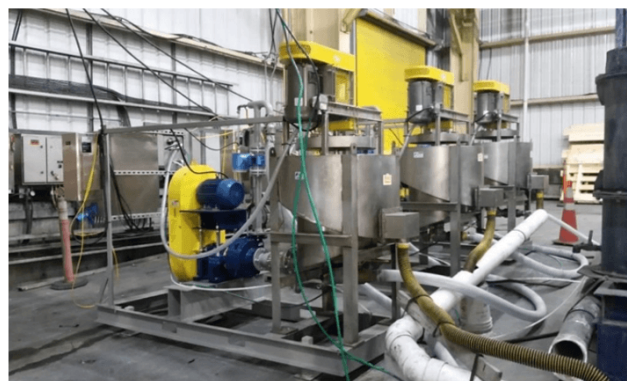
Figure 17 0.6 m diameter Stackcell used in pilot trial study for Cu-Ni concentrator
